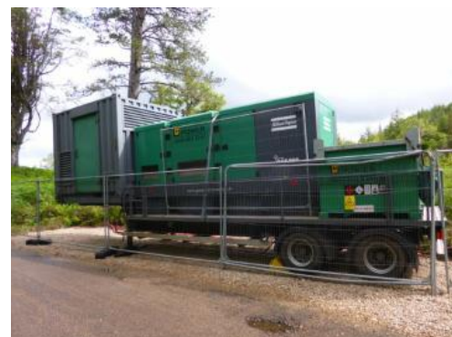
Generator at Achnacarry
