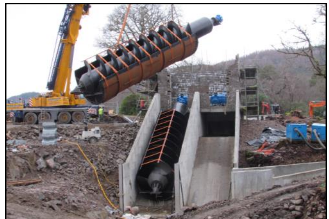
Generating Electricity on the River Arkaig Twin Archimedean screw hydropower turbines being installed on the River Arkaig. Water will be diverted from above a weir, through the turbines and reintroduced to the river 200 m downstream. The new scheme is being constructed just downstream of the existing weir.
